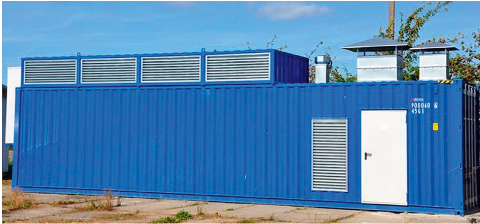
Photo 1. View of an energy storage container
